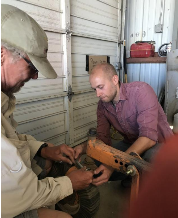
Joshua Abbe (right) confessed to parking the golf cart in a non-optimal spot, causing a Hangar 3 door roller to jump out of the track when opening the door. Here, he and John Gillis effect repairs. Pro tip: Don't park the golf cart right next to the hangar door. Photo by Becky Kinder
