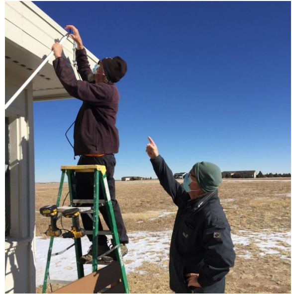
John Gillis installs the new antenna for the Open Glider Network (OGN), while Kip McClain supervises
