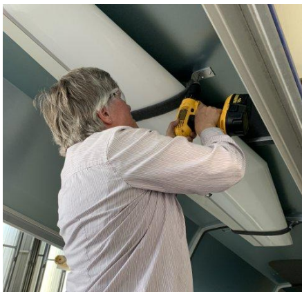
Alice Palmer works on relocating the tail holders on the Cobra trailer.
