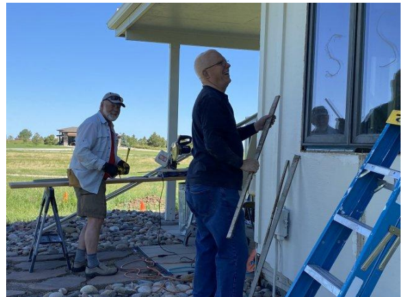
Gary Baker and Frank DeBacker work on installing the new clubhouse windows. Photo by Becky Kinder
