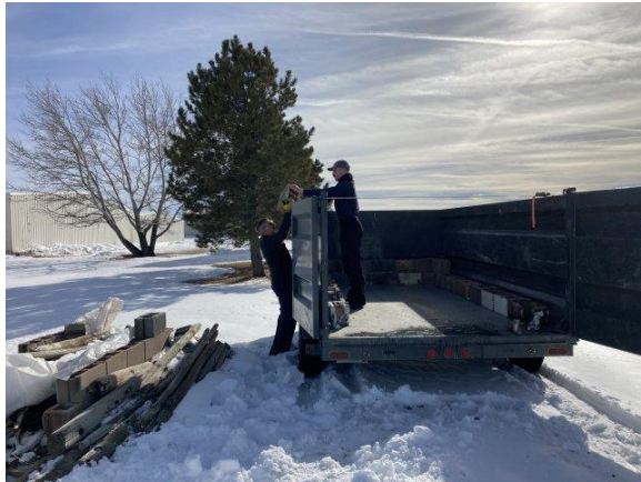
Andy, Joe, and Terri Gerner start to disassemble the old cement block fire pit.
