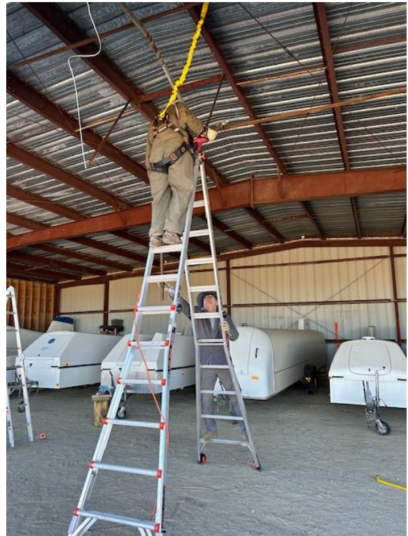
Bill Gerblick works on the hangar door project, protected by both Safety Spotter Raul Boerner and the safety harness (which, as we understand, was tested for real during this project and it worked—fortunately!).
