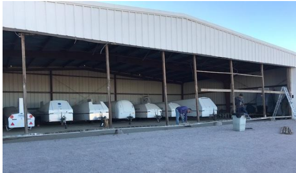
Old sheathing removed; now to get down the frame. Photo by Raul Boerner
