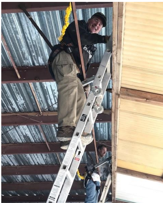
Bill Gerblich and Scott Dimick begin the demolition project on the Hangar 3 door. Photo by Raul Boerner
