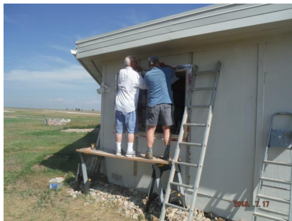
Frank DeBacker and Gary Baker installing one of the new windows (with Steve's help)
